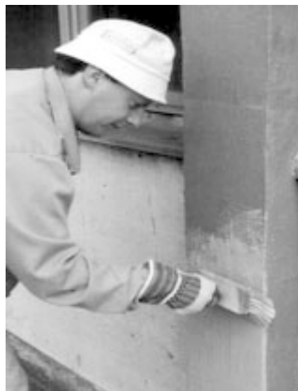
Figure 10. Typical application of a cementitious water-proofing sealing slurry by brush (Wacker Polymer Systems)
